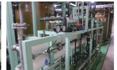
Water purification apparatus
