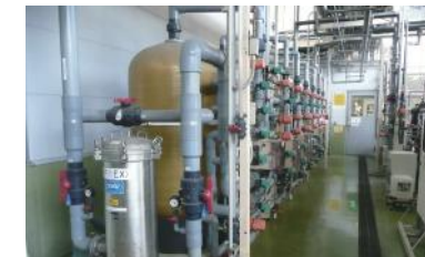
Ion exchange tower
